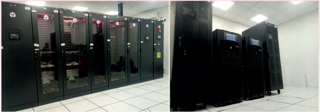
Himachal Pradesh : S-NOC Server Room
